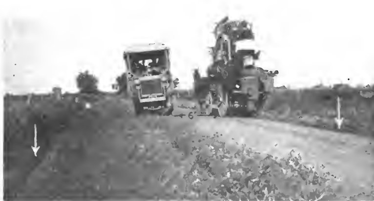
A plain dirt road good only in dry periods. There are side drains but they are heavily grown with grass and weeds along the edges of the road prevent a quick discharge of surface water. Only little work has been put onto the road, but none of it lost in trying for overwidth. That it is wide enough is shown by the positions of the two vehicles, their separation being more than needed for safe driving.
